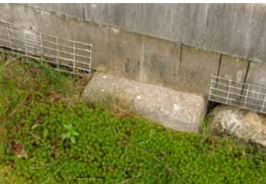
Above top: Interior dining room window. Above bottom: Shingle wall base. The foundation, which really was pretty good... considering. Very well drained soil kept it from collapsing. Photos courtesy of Knight Associates.
